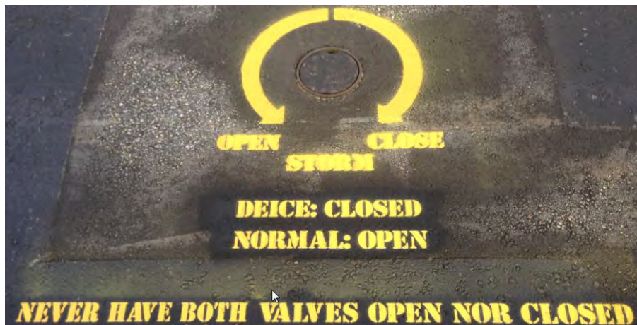
Photo 1: Stormwater gate valve and operating position indicators.
