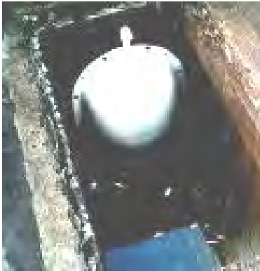
Storm Drain Hood
