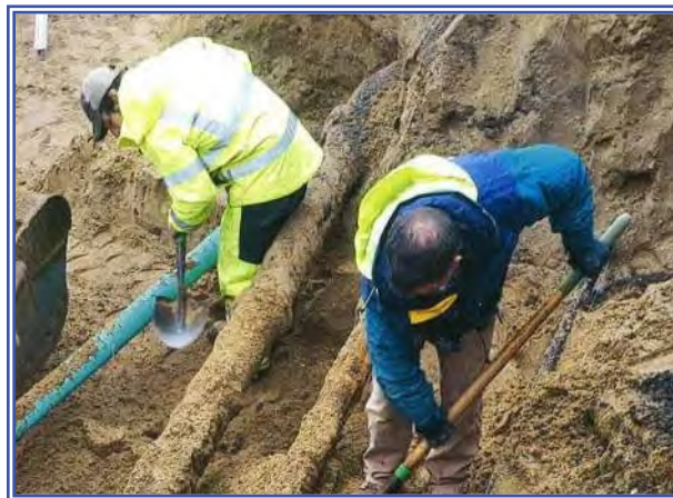
Fire Service Installation
