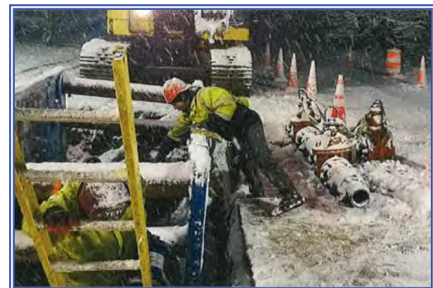
The night-time installation of a 3-way valve cluster during a snow event in Hyannis
