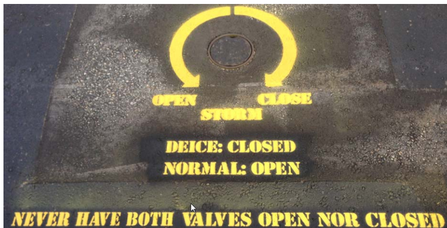
Photo 1: Stormwater gate valve and operating position indicators.
